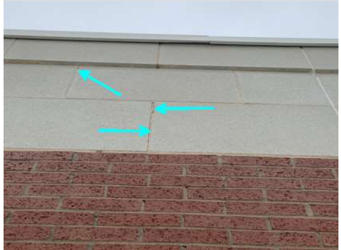
Example of cracks in stone mortar
