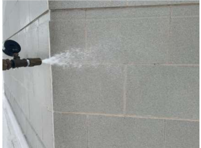
Water tests of block wall produced leakage.
