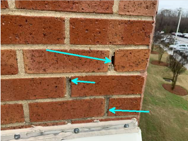
Gaps in brick above critical termination.
