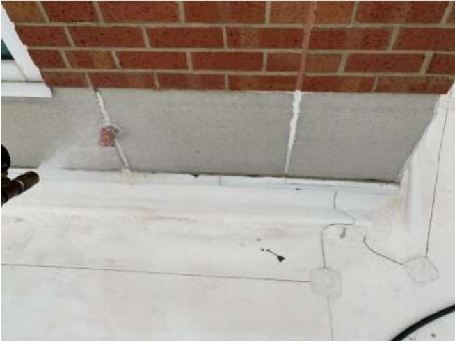
Water tests of various areas above leak area did not produce visible leakage during tests.
