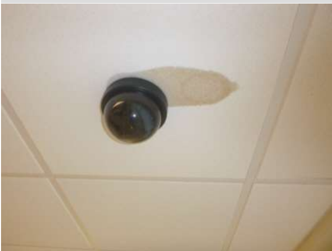
Small leak area at camera
