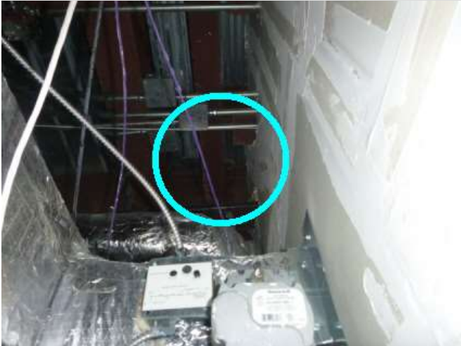
Visible leakage noted during test same area as stains and rust
