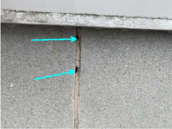
Typical crack / gap noted in stone mortar joints (area tested)
