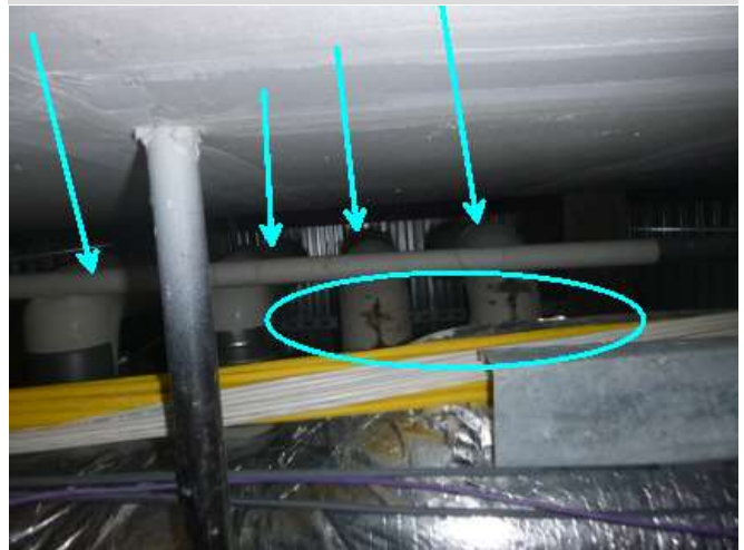
Removal of tiles showed pipe penetrations at 2nd floor (arrows). Visible leakage (circle).
