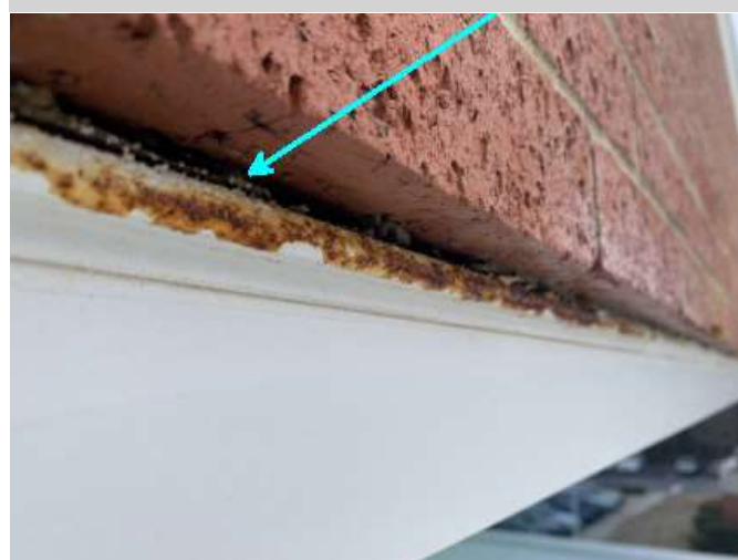
Close up of brick angle ledge above windows - test of upper side of angle produced leakage
