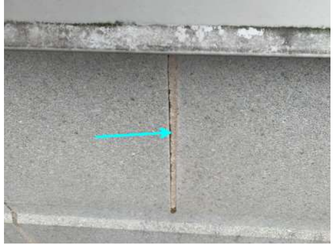
Typical crack block mortar
