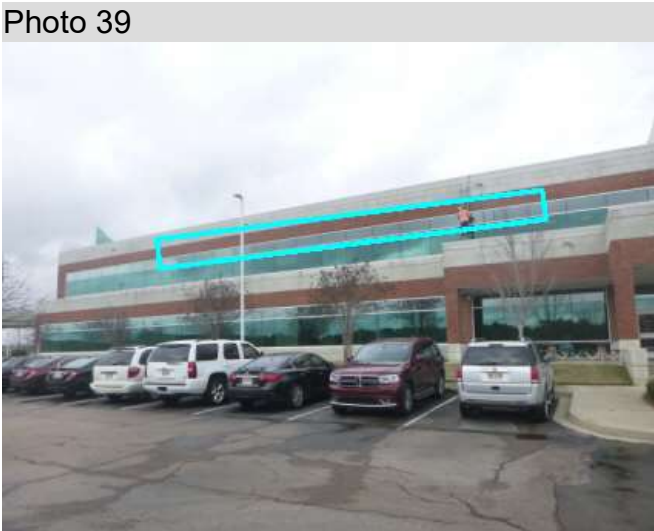
Leak area #3 - leakage at tops of various administrative office windows.
