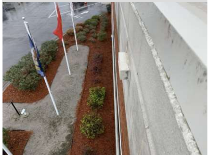
Exterior of Leak area #7
