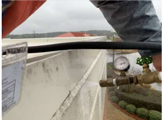
Water test of gaps in the exterior block wall below coping produced leakage in exact location of interior.
