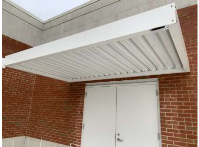
Mechanical Room directly above Leak area 1 Awning has been installed
