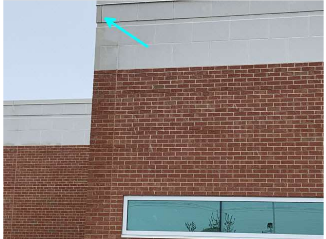
Large gap in stone mortar joint noted at corner
