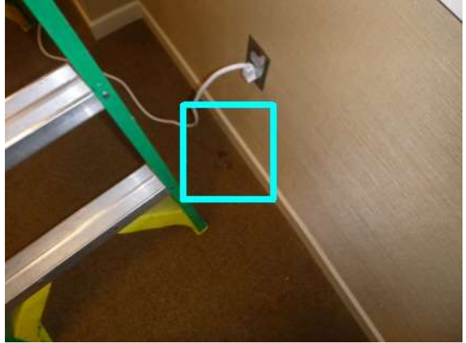
Water dripping onto floor during testing.
