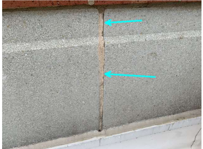
Cracks in nearby stone mortar joints
