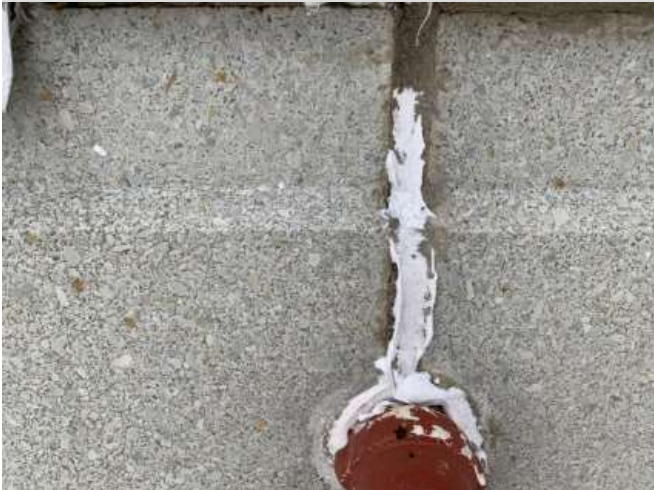
Previous repair attempts with sealants (not professional application)
