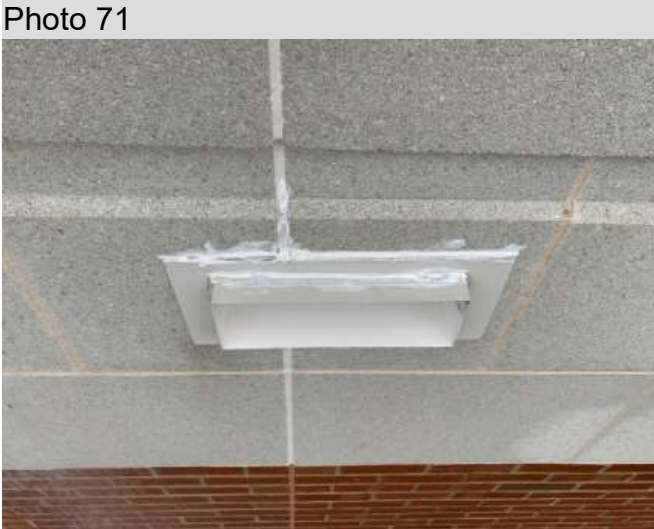
Close up of scupper shows unprofessional sealant application
