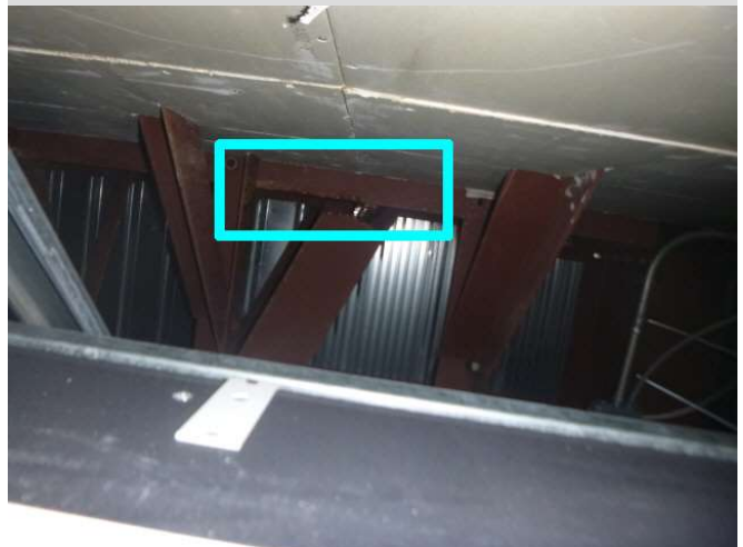
Water leaking in this area during testing
