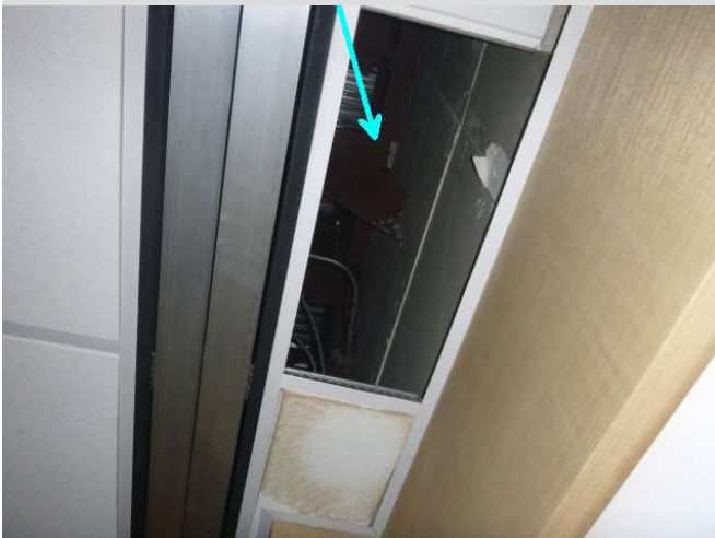
Leakage during test at transition
