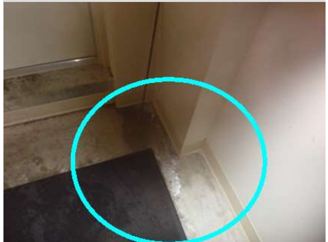
Leakage spread across floor and leaked into admin ceiling area below.
