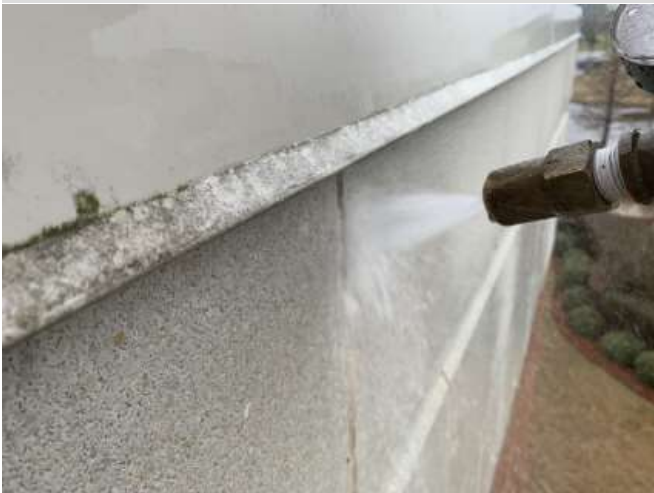
Water test of mortar gaps / cracks produced reported leak.
