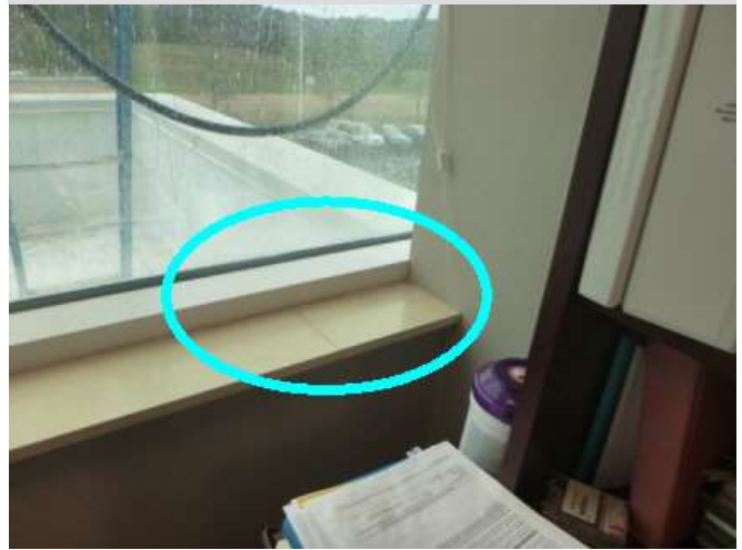
Water ponds at window sills.
