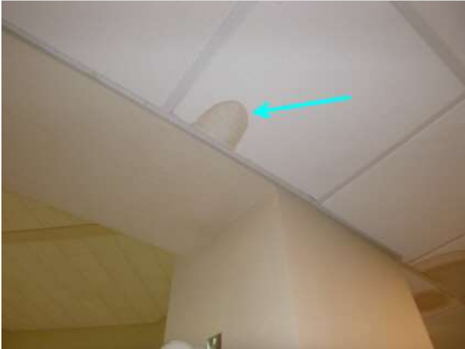
Water stain at north side of column
