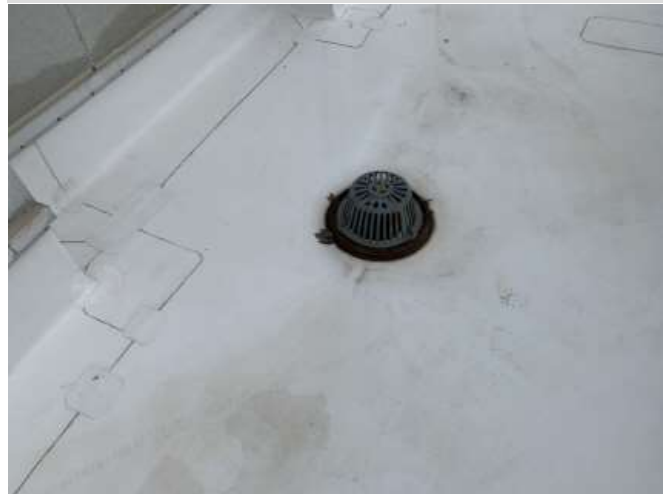
Roof drain directly above stain in front entryway
