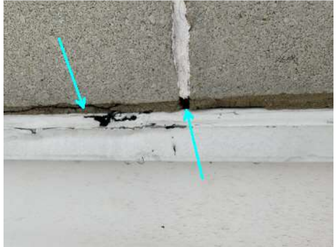
Gaps and cracks note in mortar
