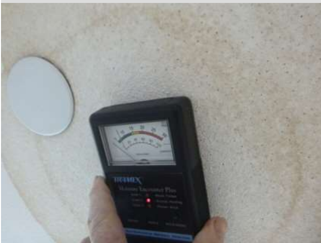
Moisture scan of water stain shows area is currently dry.
