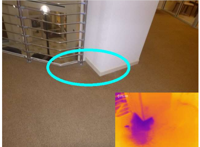
Wet carpet at base of column. Infra red (bottom right) shows wet.
