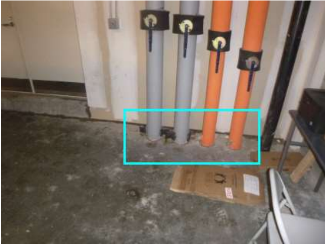
Pipe penetrations above leak area. Leakage noted through penetrations below.
