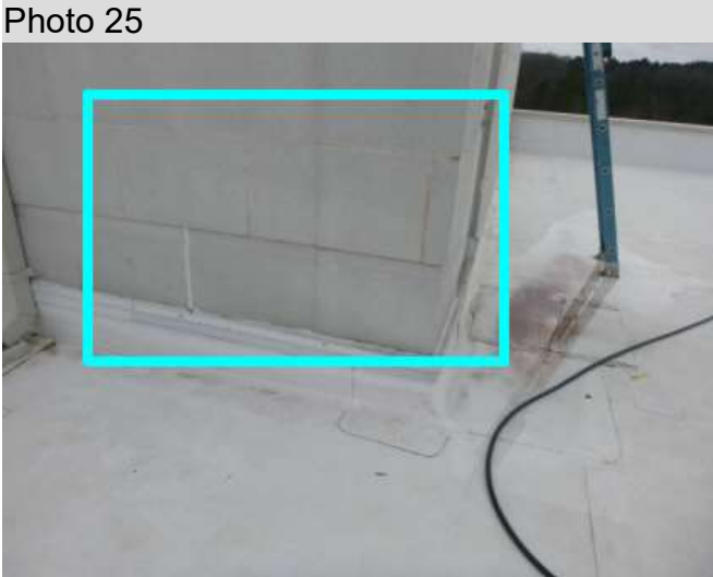
Water tests of mortar joints gaps and cracks in stone produced the reported leakage
