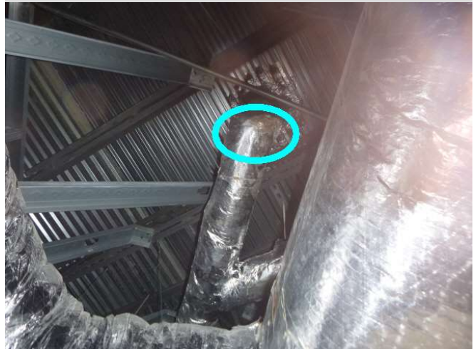
Elbow in roof drain directly above stain in entryway
