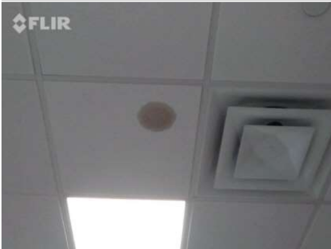
New water stain noted below drain in front entryway
