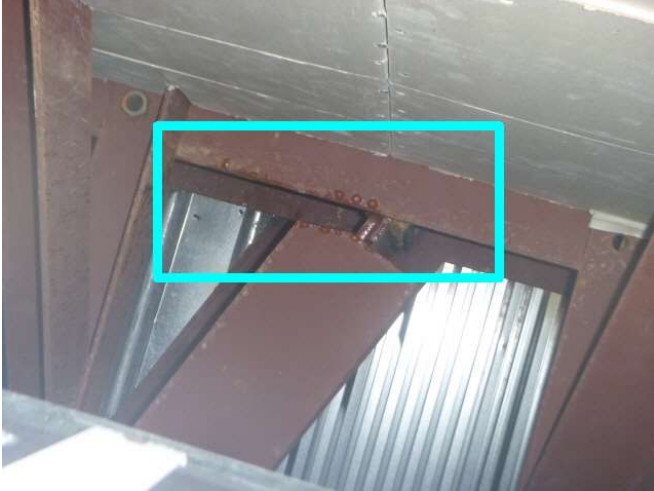
Visible water dripping during test
