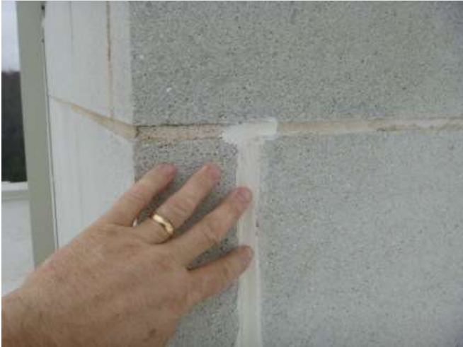
Example of sealants used in attempt to seal crack in stone mortar joint
