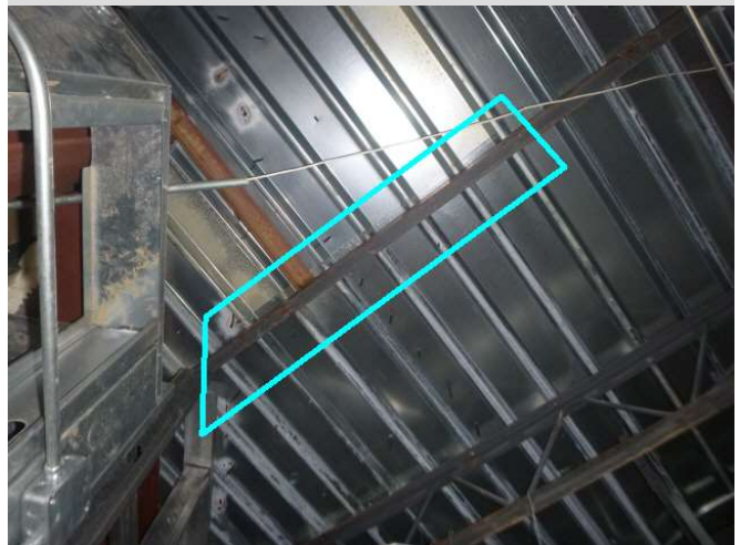
Leaks produced between seams of roof decks in area directly below wall during tests.
