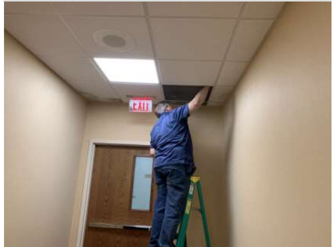
Inspection of area above ceiling shows water stains and rust stains.
