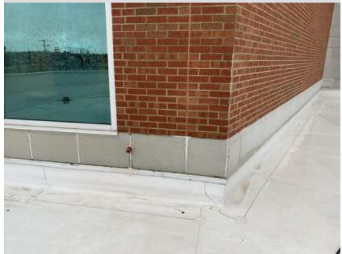
Exterior directly above leak area
