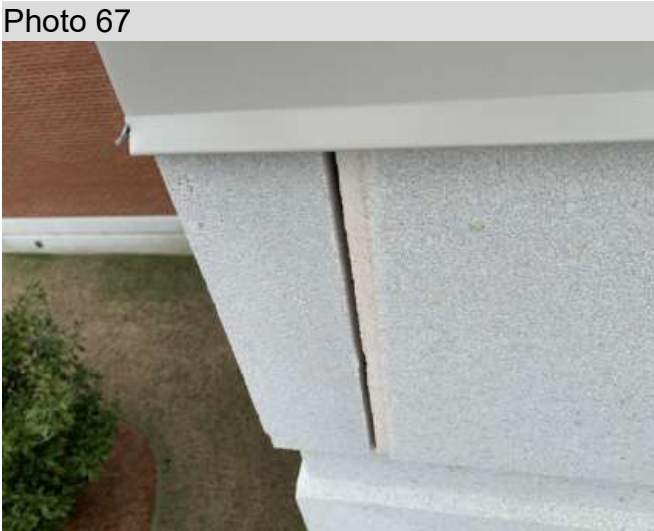
Closeup of large gap above the leak area in the corner interview room
