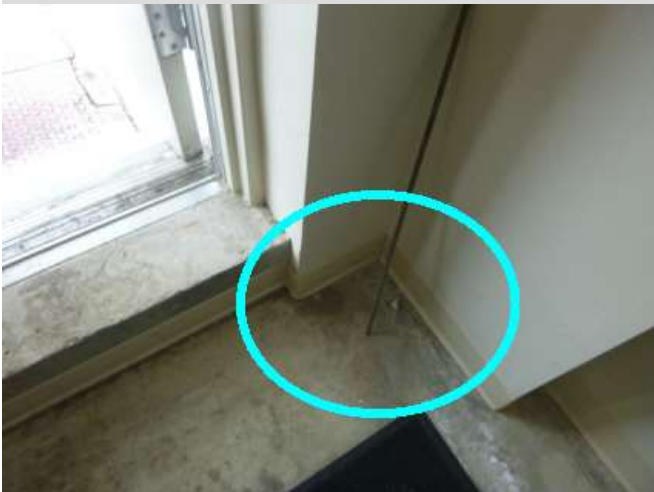
Leakage onto stairwell floor noted.
