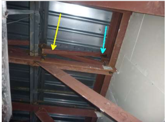
Small leak came in at exterior wall roof deck juncture (blue) and ran down the angle iron cross brace and drip to exact area of stain (yellow). Note active water trail visible.
