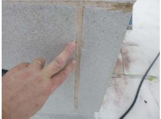
Example of crack in mortar joint - many noted like this. Can cause capillary suction into wall cavity
