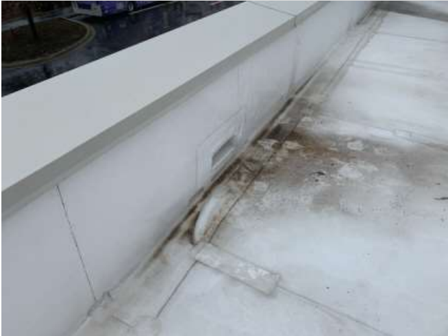
Test of roof area and coping above leak area did not produce any visible leakage
