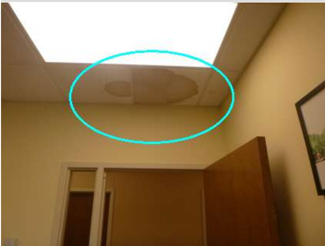
Wet ceiling tiles inside office
