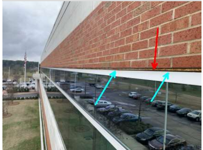
Noted missing sealants at bottom of angle ledger (blue arrows). Angle iron itself shows some rusting (red)
