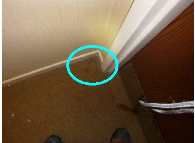
Water dripping onto carpet during test - same area as stain on ceiling tile.
