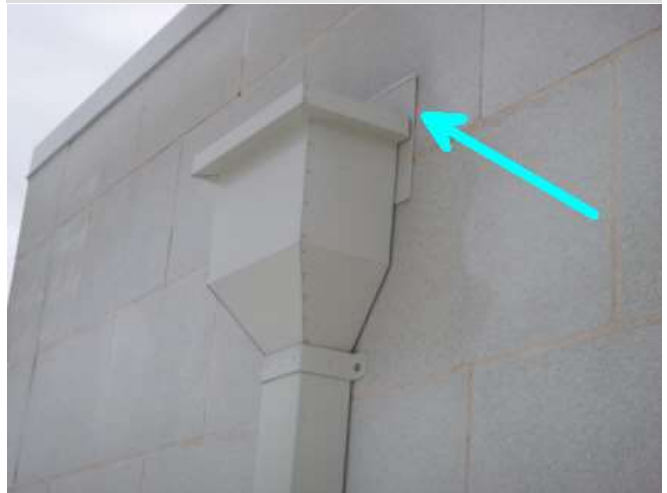
Sealants at ALL scupper catch box details and face plates should be professionally resealed to help prevent water intrusion into wall cavity.
